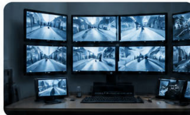
8 Security monitoring systems
